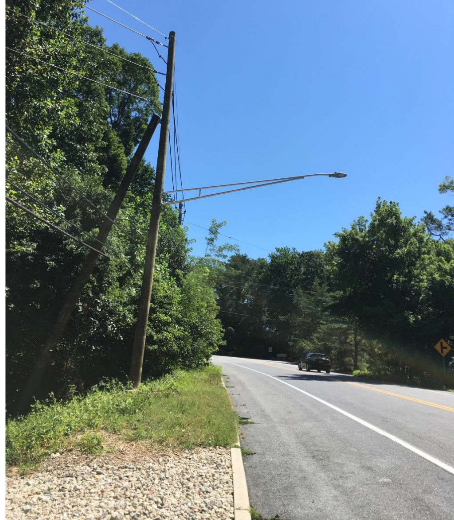
Photo 2 – Street light relocated to the new utility pole along West Benfield Road.
