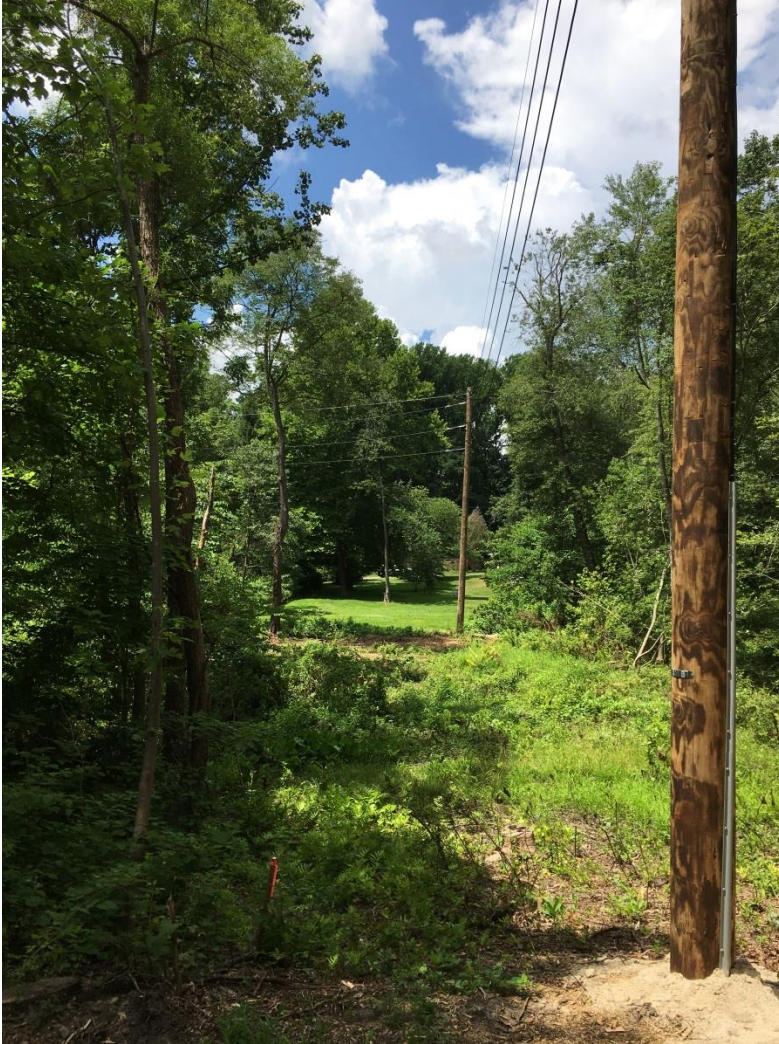
Photo 1 – New poles installed by BGE and electric lines relocated north of West Benfield Road.
