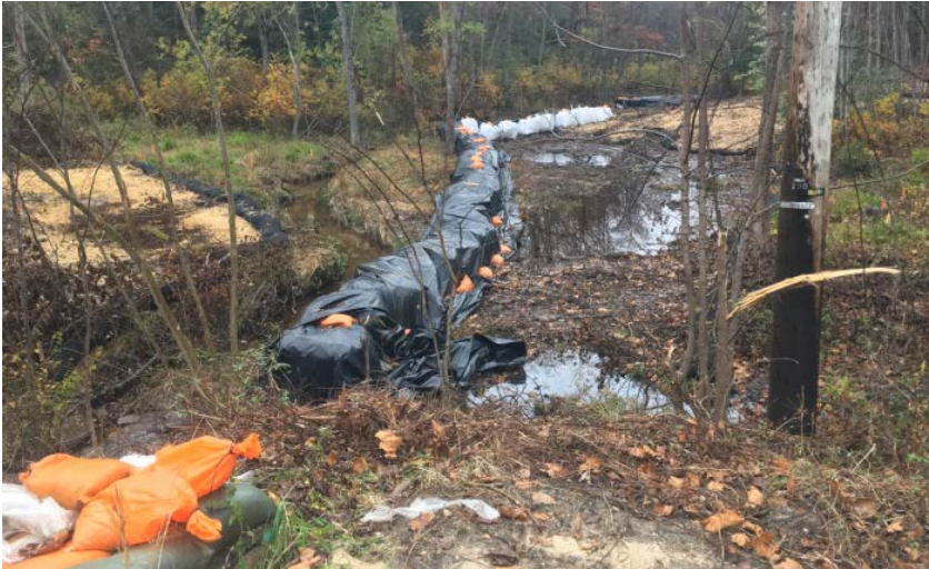
Photo 1 – Utility Pole blocking installation of diversion channel & pipe
